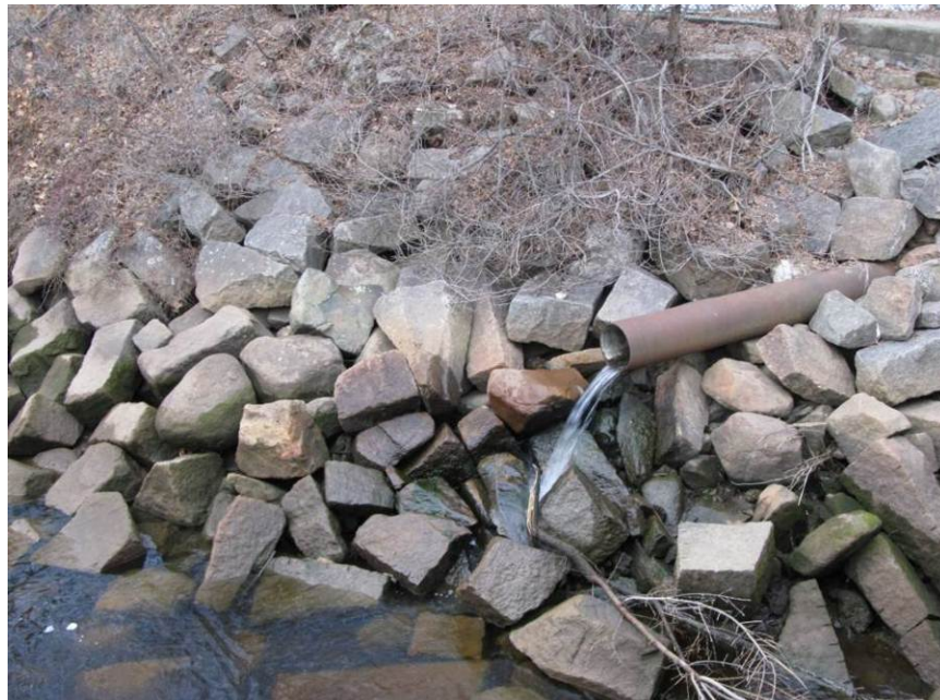
Figure 22: Stormwater discharge through drainage pipe adjacent to the Shaw Street Bridge. Photo by Benjamin D'Agostino.
