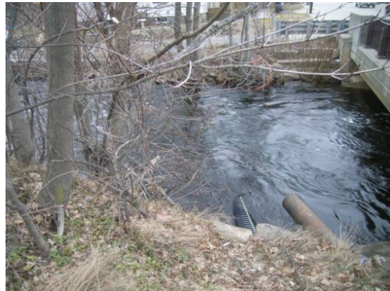
Figure 62: Point discharge adjacent to Adams Street Bridge. Photo by Eddie Haynes
